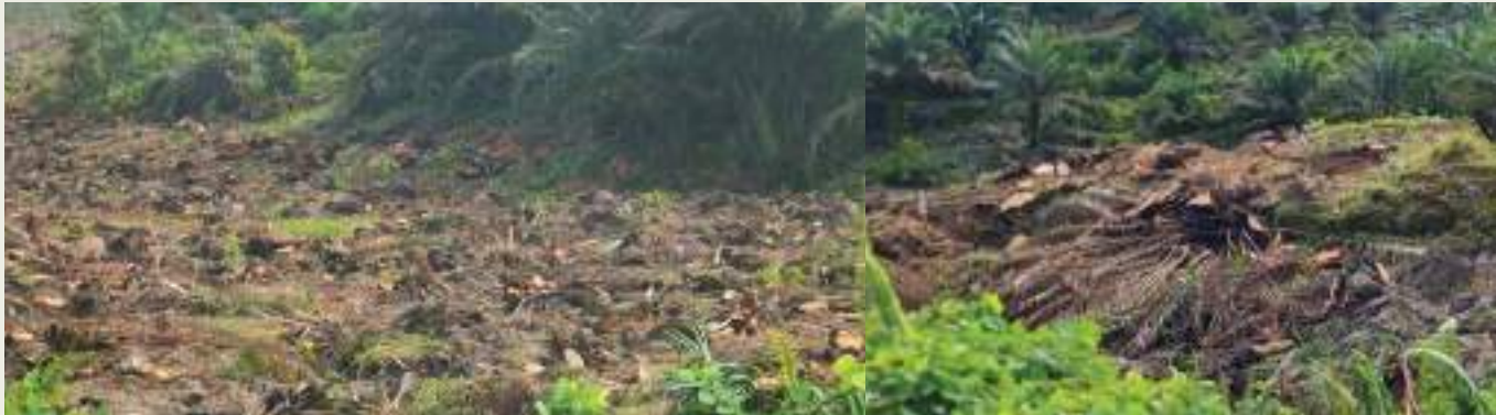
Zero burning. Practice of felling, chipping and stacking implemented at replanting areas
