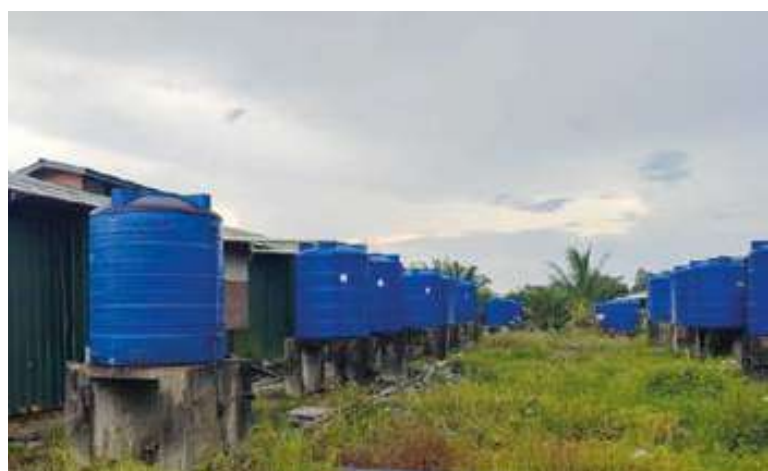
Rain water harvesting tanks
